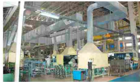
Air cooling of welding shop with fumes exhaust
